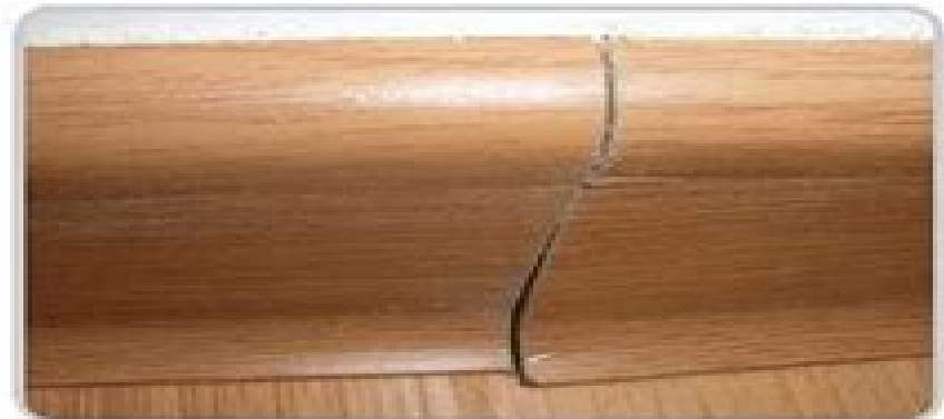
Skirting line cracks
