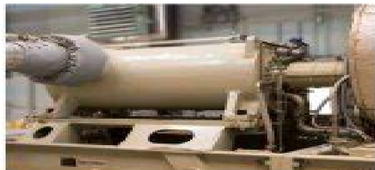
C61 Gas Compressor
